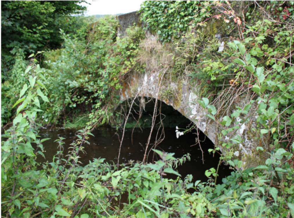
Photo 58 - Single arch masonry bridge on Arrigle River at Grid Ref S 607 322. No bats roosting in structure
