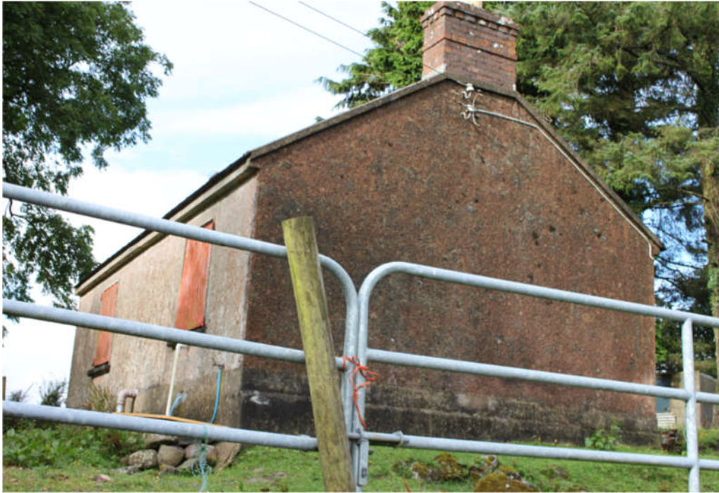
Photo 52 - Dawn survey conducted at derelict cottage Derrylackey Lane. (Grid Ref S59179 28552). No bats returned at dawn
