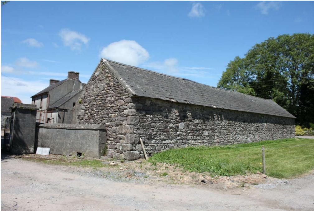
Photo 34 - Northern farmyard on Castlebanny Lane (Grid Ref S56754 32266) comprising derelict farmhouse and stone outbuildings with slate roofs. View from Castlebanny Lane.
