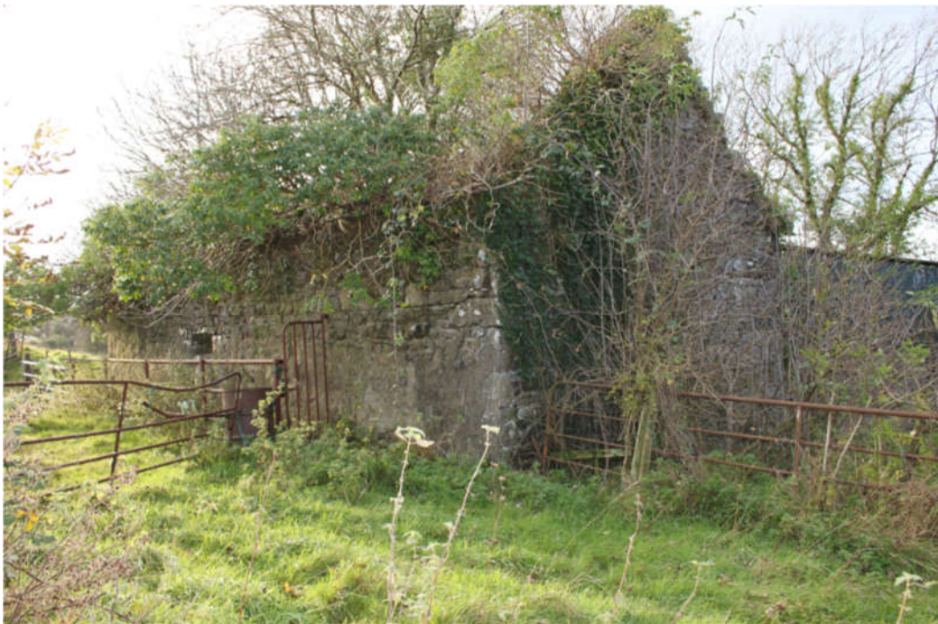
Ruined stone farm building on Castlecosker Lane. A lot of activity of Brown long eared bats was recorded on a remote bat detector in the vicinity of this building. It most likely contains a roost of Brown long-eared bats. An emergence count will be conducted in May 2108.
