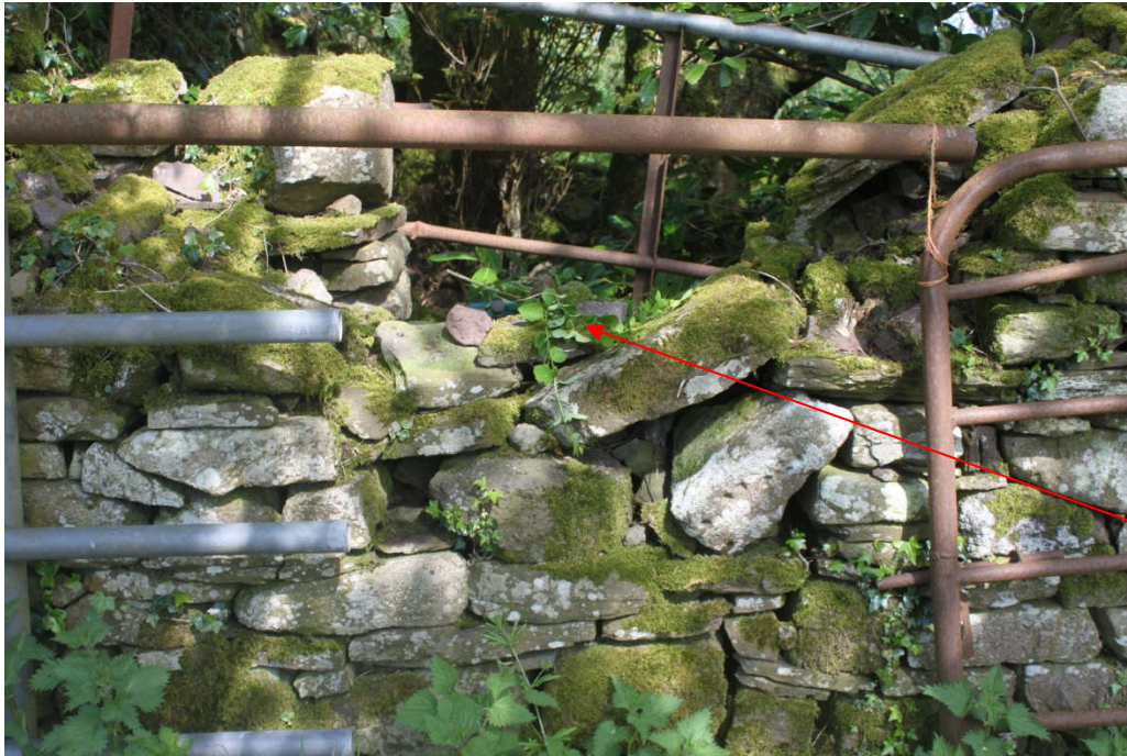
Photo 28 - Stone ruins on lane to northern mast (S56883 33360). Position of Songmeter SM2 is indicated on wall to rear of building
