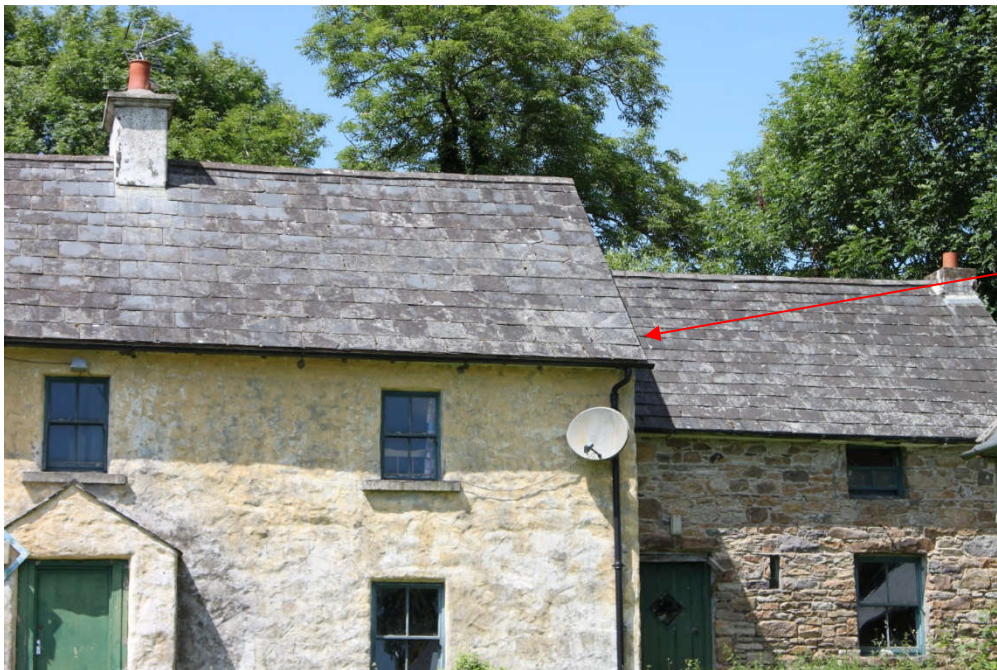
Photo 39 - Two storey farmhouse at Coolroebeeg Townland. The exit point from the roost space in the attic is indicated.
