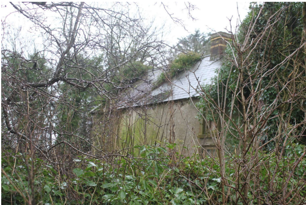
Photo 49 - Dawn survey conducted at derelict farmhouse for sale just north of Castlebanny Lane. (Grid Reference S56030 32592). No bats emerged.
